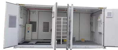
1075KW HH ESS
