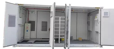
1075KW HH ESS
