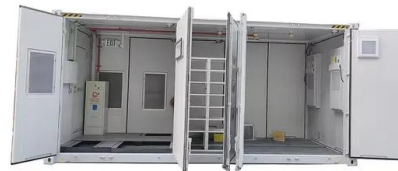
1075KW HH ESS
